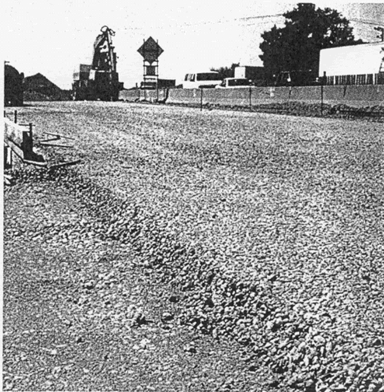
This sub-base material is cement coated aggregate. Extremely water permeable and strong, the material is place with an asphalt paver.
