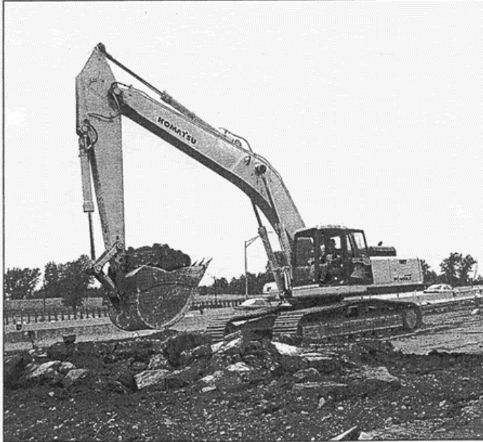
Operator Mike Fintak is excavating existing pavement with a Komatsu PC400 excavator rented from Rupp Rental/Anderson Equipment Company.
